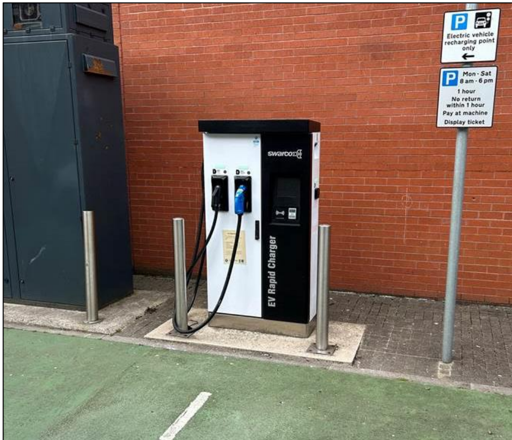
New EV Charger in Mill Street, Perth
